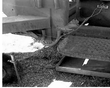
Figure 8-2. Generator improperly grounded
